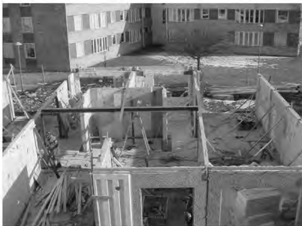
Figure 4. Frame construction in Nya Udden. Additional steel supports were used to further reinforce the building.
