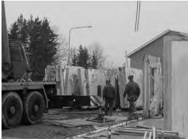
Figure 3. The concrete elements from the refurbishment project arrived at the building site in Linköping, Sweden.
